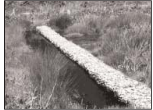
Reedbed inlet structure. Stone-filled gabions filter and slow water into the reedbeds. Courtesy of Munro + Whitten
